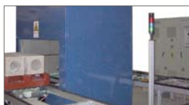
Production Line with a 30kW Microwave Chamber Oven for Drying Ceramic Blocks
